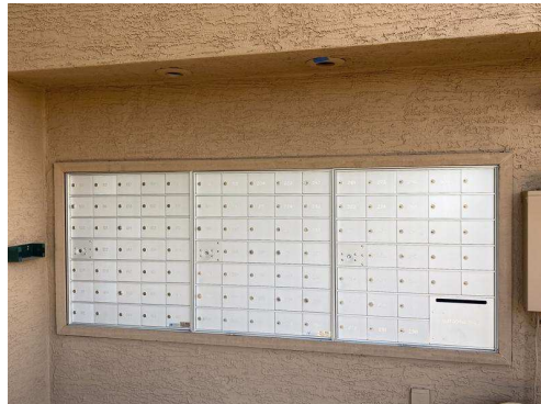
Good condition. (3) 5 x 7 cluster box sets covered. Replaced in 2017.
