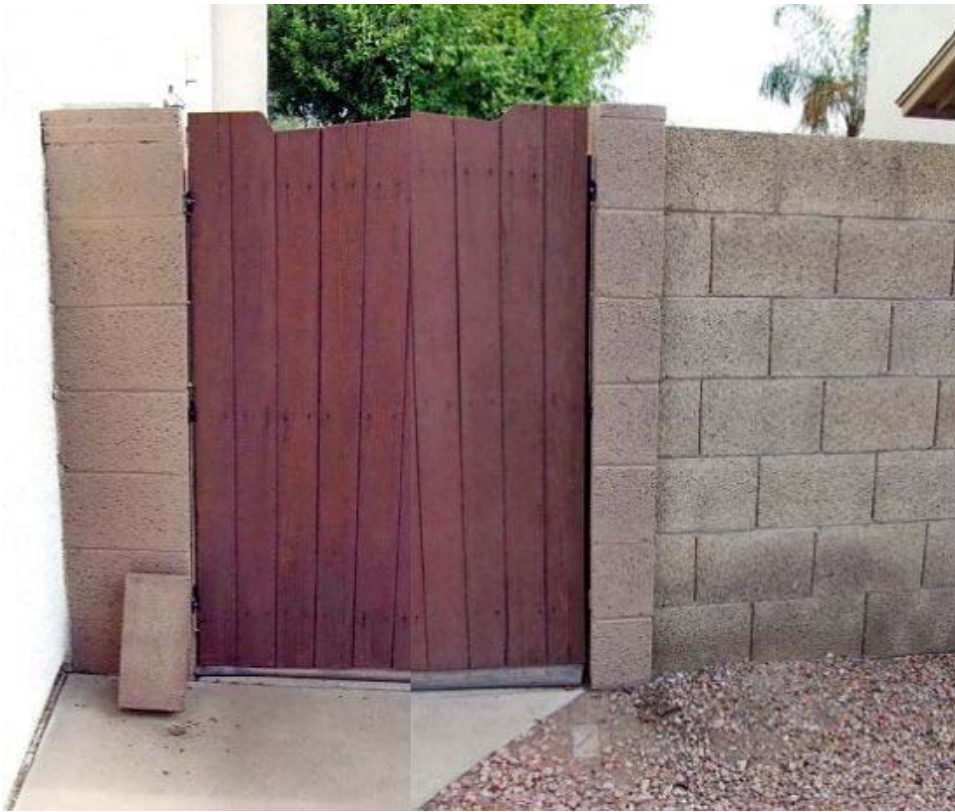
Gate with painted block next to stained unpainted wall.
