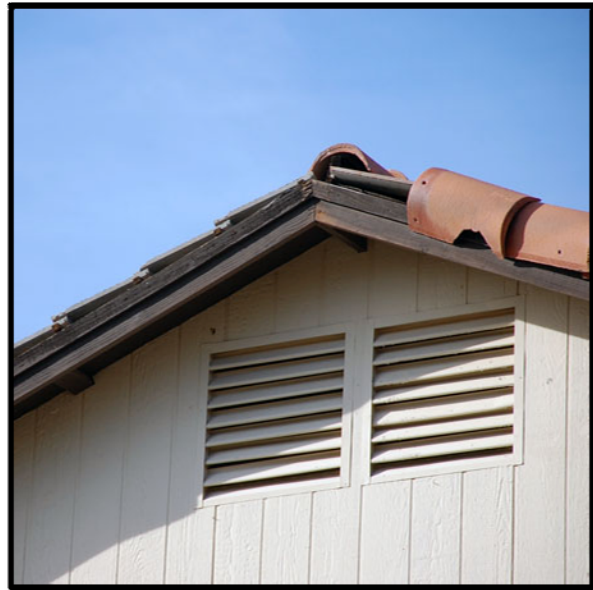
Tiles Need Replacement
