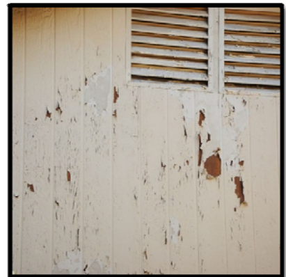
Wood Trim In Need of Repair
