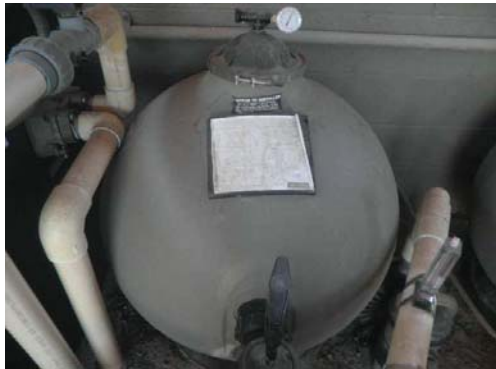
Hayward sand filter S311SKV. Sand replaced and repairs 6/2017.
