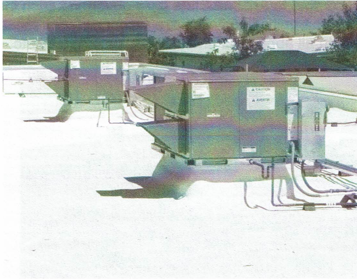
Figure 2 – Typical result of an approved method of a new Air conditioning unit's installation using an 8-inch mounting curb
