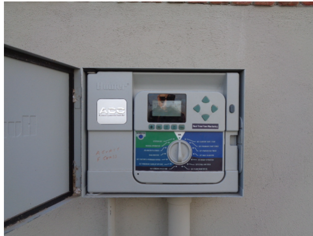
This is a Hunter ACC-99D controller located at the entrance to the community.
