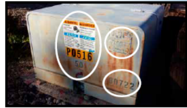
Do not paint over stenciled information or reflective stickers on instructional and warning decals (see circled examples above).
