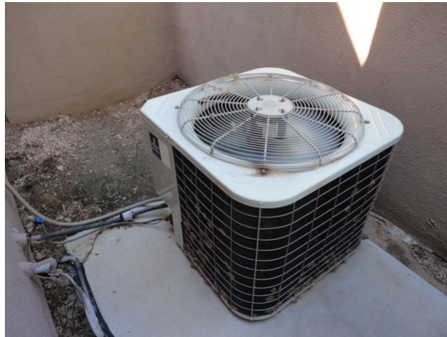
Rheem, 3.5 ton split system w/heat pump (replaced in late 2018 at a cost of $6,528.00).
