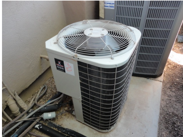
This is a Bryant, 2.5 ton split system. The useful life adjustment was provided by the client.
