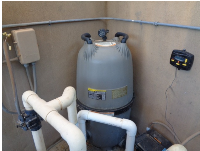
This is a Jandy CL580, 500 sq. ft. cartridge filter that was purchased/installed in mid-2021 at a cost of $1,834.50.
