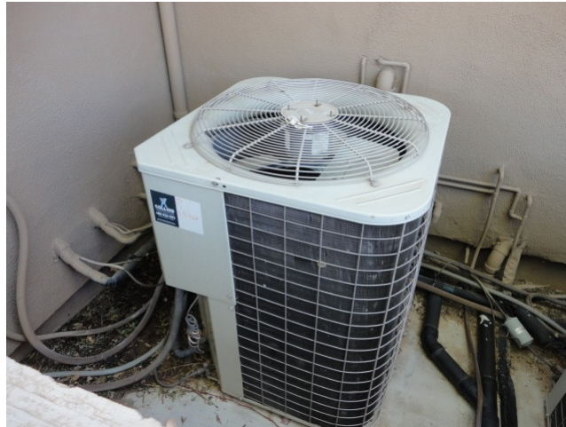
This is a Bryant, 4 ton split system. The useful life adjustment was provided by the client.
