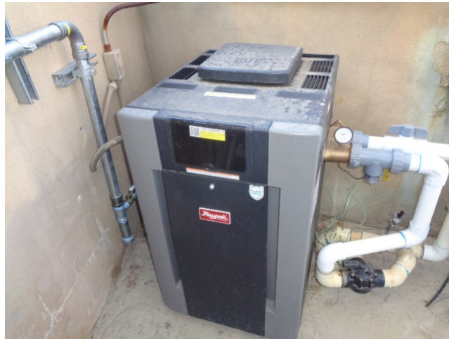
This is a Raypak, 266,000 BTU input heater (purchased/installed in July 2023 at a cost for $4,103.61).
