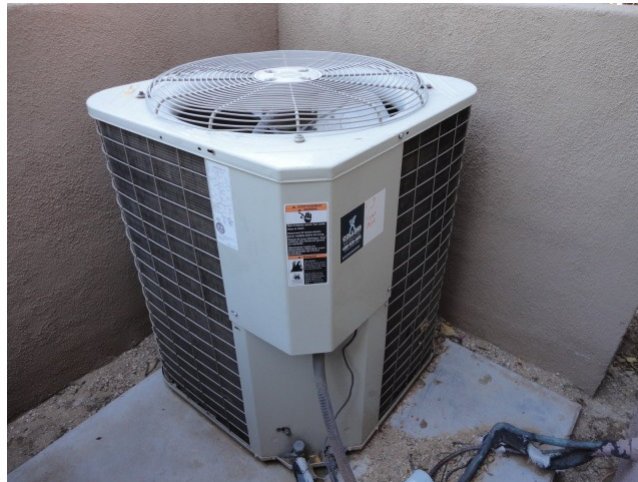
Rheem, 5 ton split system w/heat pump (replaced in late 2018 at a cost of $6,736.00).
