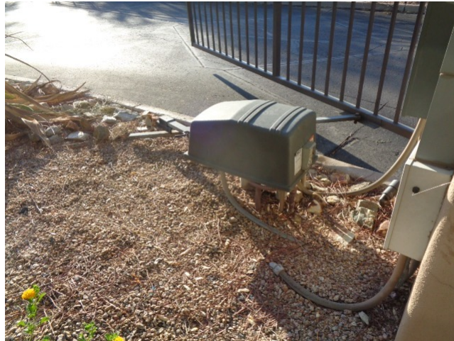
These are Door King, swing gate operators. The useful life adjustment was provided by the client.
