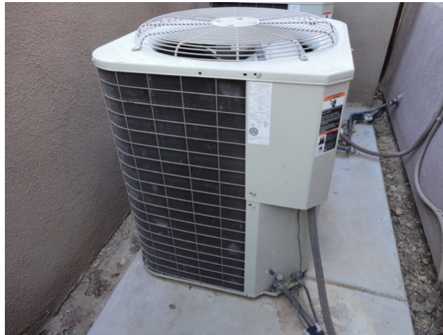
Rheem, 5 ton split system w/heat pump (replaced in late 2018 at a cost of $6,736.00).
