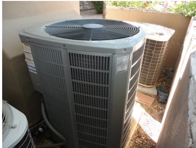
American Standard, 5 ton split system (installed August 2016).
