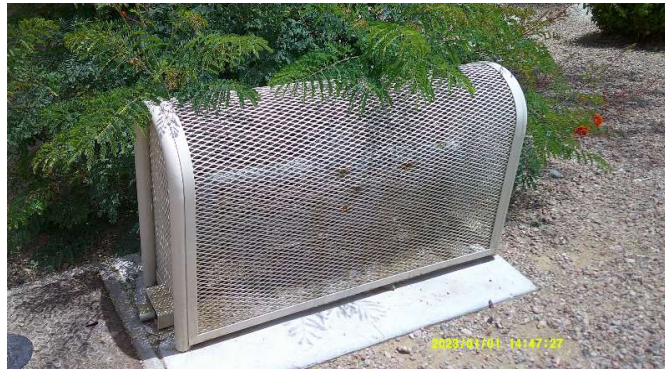
Febco 1" 825 backflow preventers. Appear to be in good condition. Cages added 2020.
