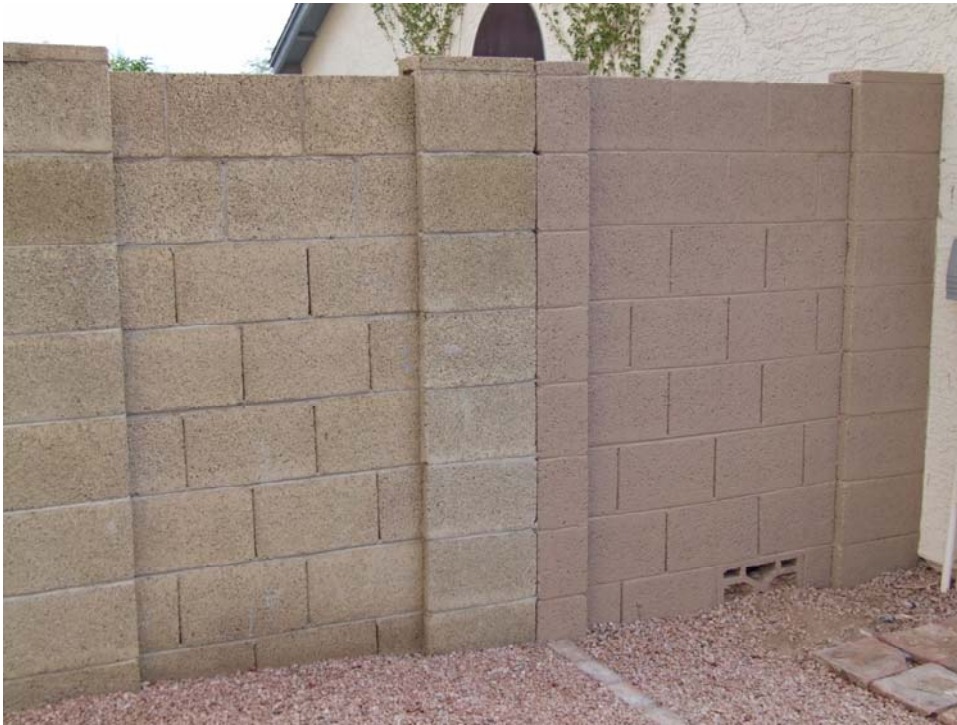
Wall (right) with painted block next to stained unpainted wall.
