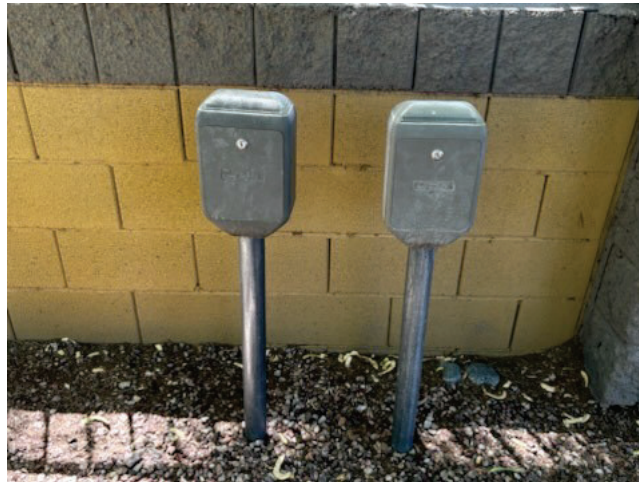
These are Leit solar controllers located next to the pool area.
