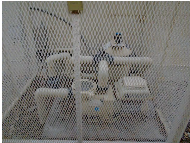
This is a Pentair, Superflo VST 1.5HP pump/motor (manufactured 4/4/2021).
