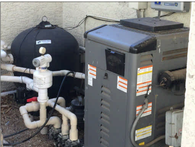
Filter, Pump and Heater
