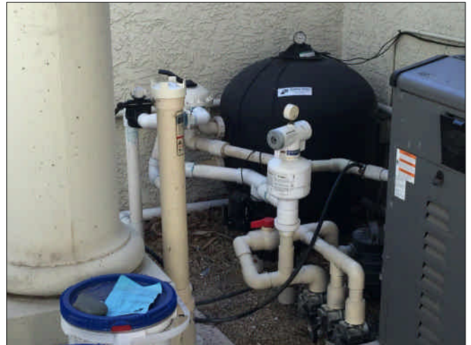
Pool Filter and Pump
